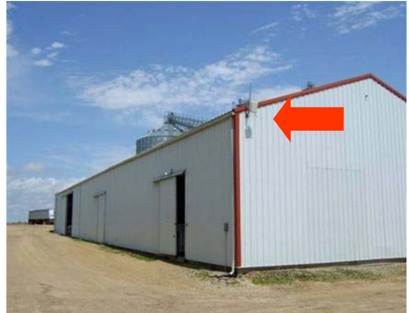
Wireless antenna installed on warehouse
